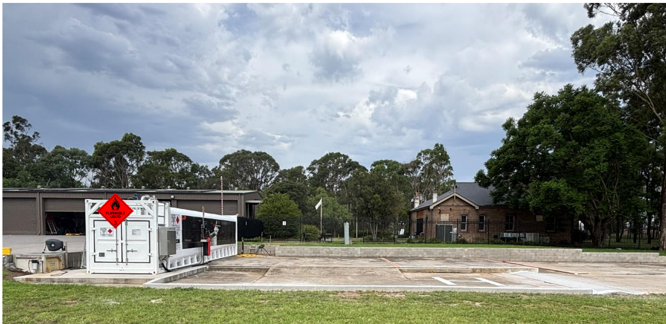
Above ground Jet A1 tank and bunded truck filling area looking east
