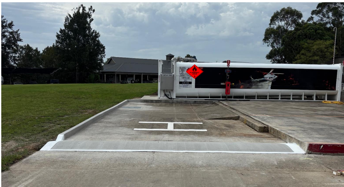
Above ground Jet A1 tank and bunded truck filling area looking north
